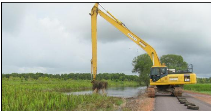
The open water areas of Fogg and Harrison Dams are threatened by growth of aquatic vegetation. Sections of Fogg Dam have been cleared to remove aquatic vegetation
